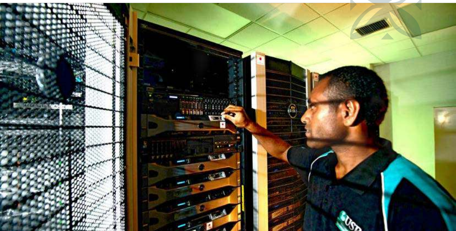
An ITS Technician inspects one of the USP servers
